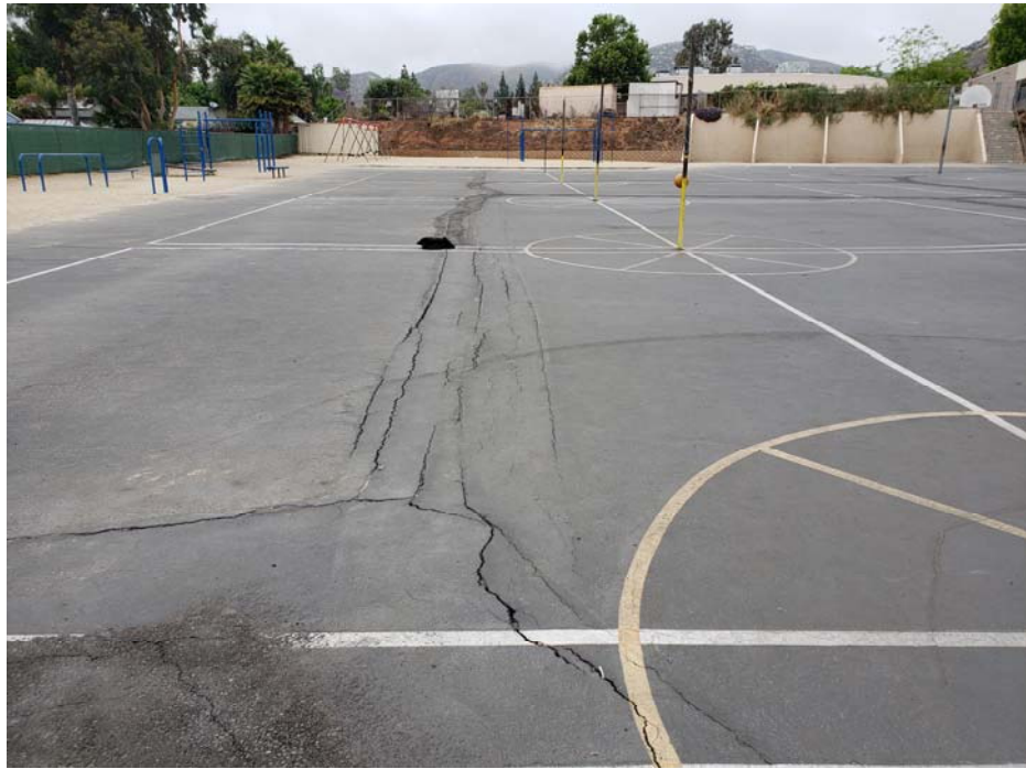
Photograph 1: View of hardcourt play area looking north. Open cracks running in the north-south orientation.
