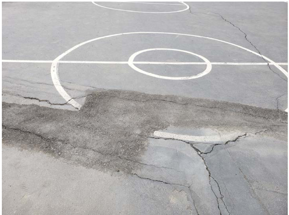
Photograph 4: Close-up view of open cracks and cracks previously patched and since reopened.
