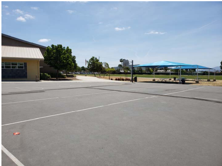
Photograph 2: View of hardcourt play area looking southeast. Patched cracks running in the north-south and east-west orientations.
